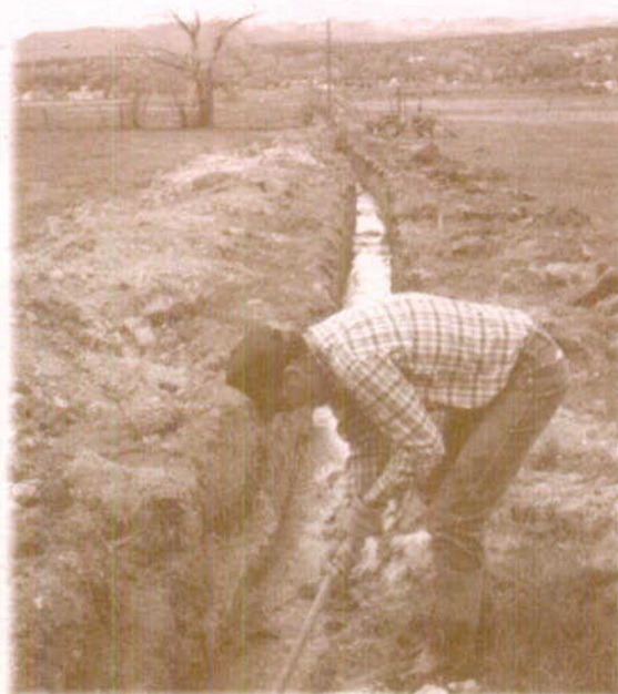
Wrights Mesa rancher lays pipe to conserve agricultural water. Photo by Debra Smith
