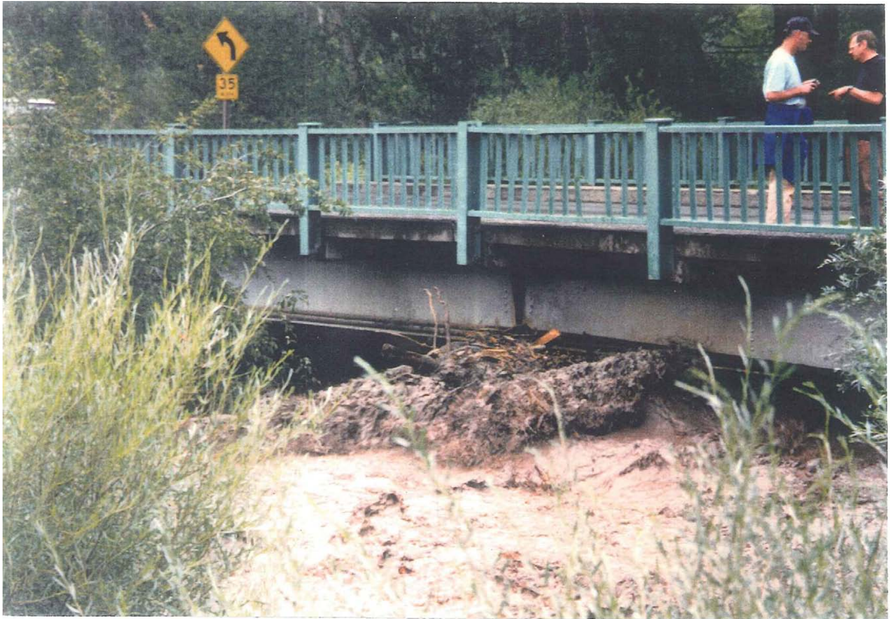
Saturday, July 31, 1999, Leopard Creek flood waters at the intersection of state highway 62 and 145, Placerville. First response personnel Undersheriff Sky Walters and Placerville fireman Gary Whitfield on right.
